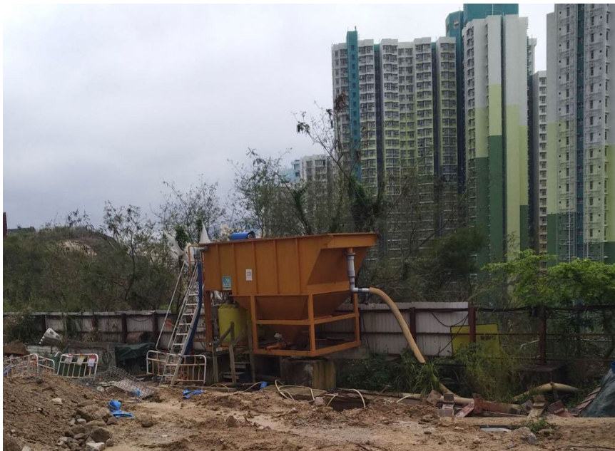
Q1. Wastewater treatment facility 30 cu.m Sedimentation Tank + AquaSed of 15 cu.m per hour + WETSEP
