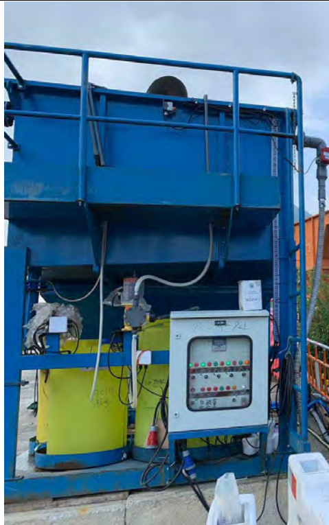
Q1. Wastewater treatment facility 30 cu.m Sedimentation Tank + AquaSed of 15 cu.m per hour + WETSEP
